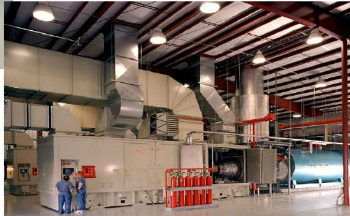
15 MW Gas Turbine Ethanol Plant
