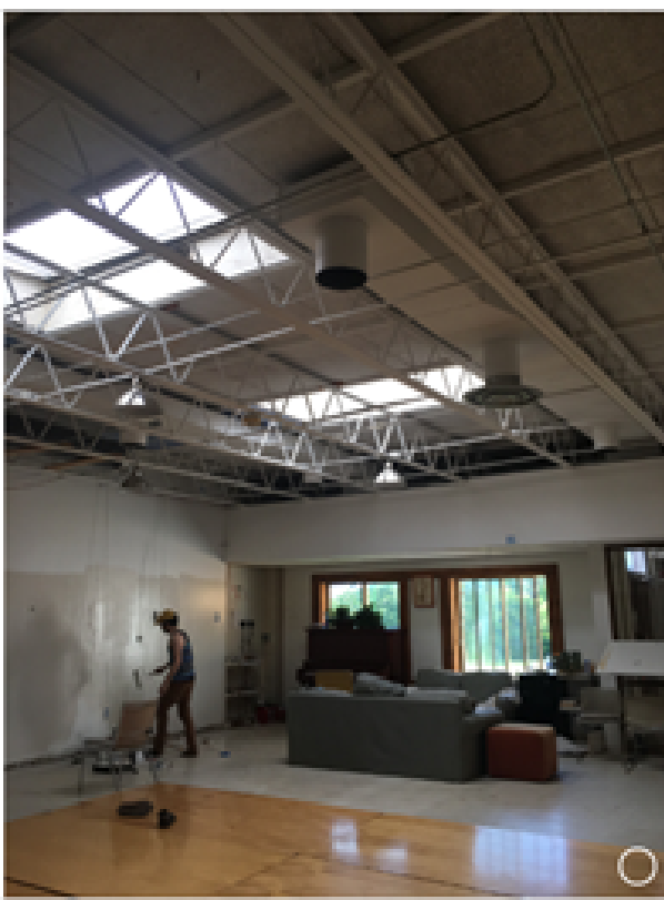
There are no working lights in this room.
